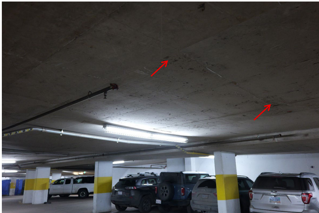
Photographs 53 and 54 show Location 27 , where concrete honeycombing was visible on the slab soffit.
