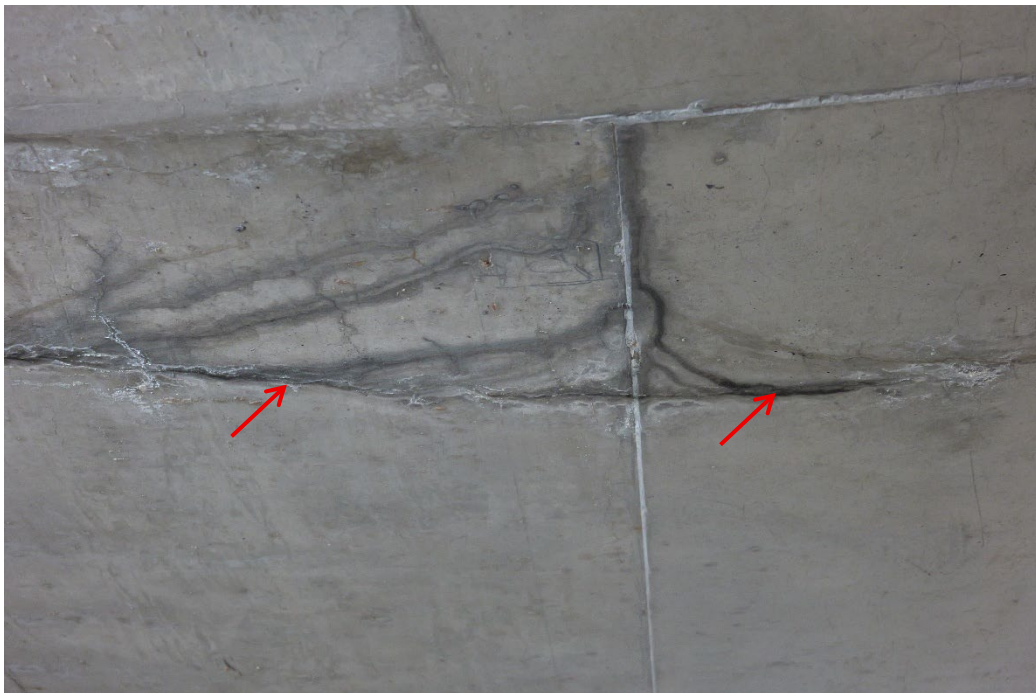
Photographs 3 and 4 show conditions at Location 2 , where crisscrossing cracks are visible in the ceiling slab. Evidence of possible leakage through a construction joint, along with associated efflorescence, is also present. Localized patch repairs are visible. 22 Station
