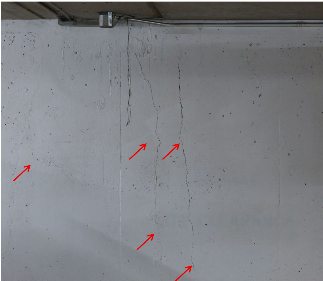
Photographs 69 and 70 show Location 35 , where cracking was visible in the retaining wall.
