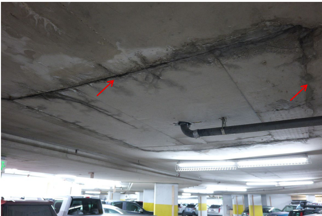
Photographs 55 and 56 show Location 28, Water leak along slab joints.
