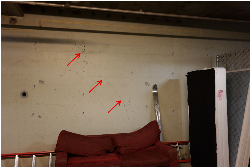
Photographs 81 and 82 show Location 41 , where honeycombing was visible on the soffit, and cracking was visible on the wall. 22 station
