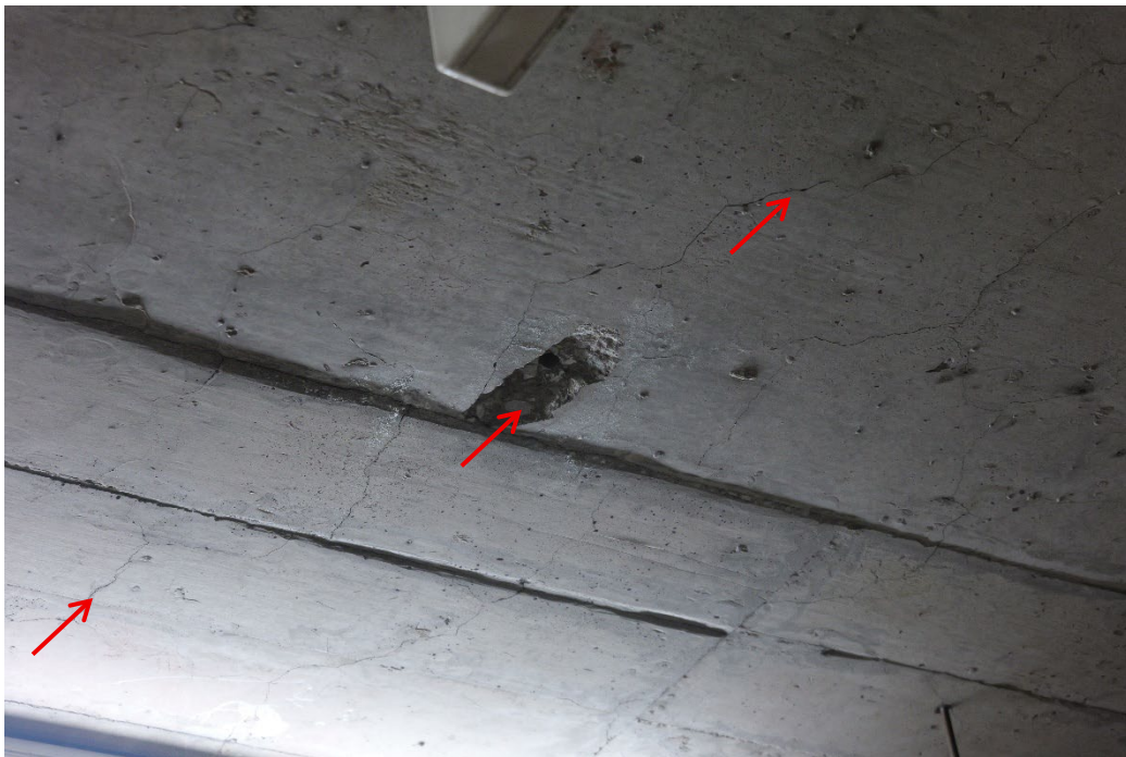
Photographs 1 and 2 show crisscrossing cracking in the ceiling slab at Location #1 . Efflorescence and localized spalling were observed. 22 Station
