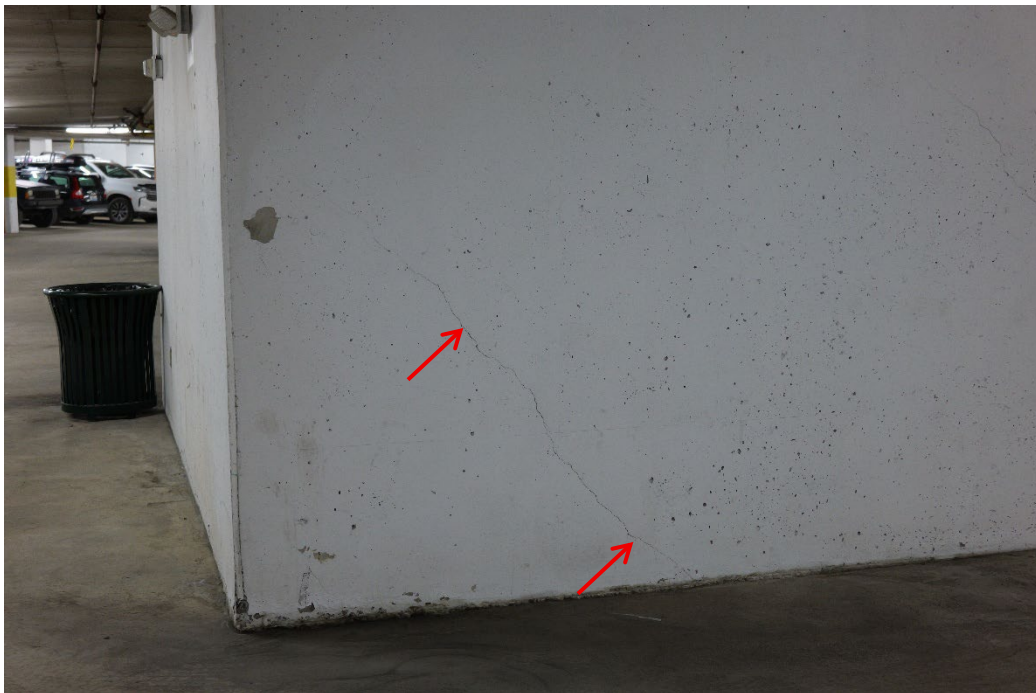
Photographs 63 and 64 show Location 32 , where cracks radiate from pipe openings and localized slab honeycombing is visible. A diagonal crack was also present in the staircase wall.
